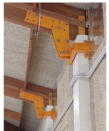
Greerton Seismic brackets
